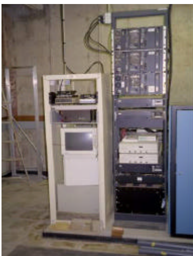
To the left, our equipment bay in the secured building at the base of the tower. The new 7/8ths inch heliax was routed to the top of the cabinet.
