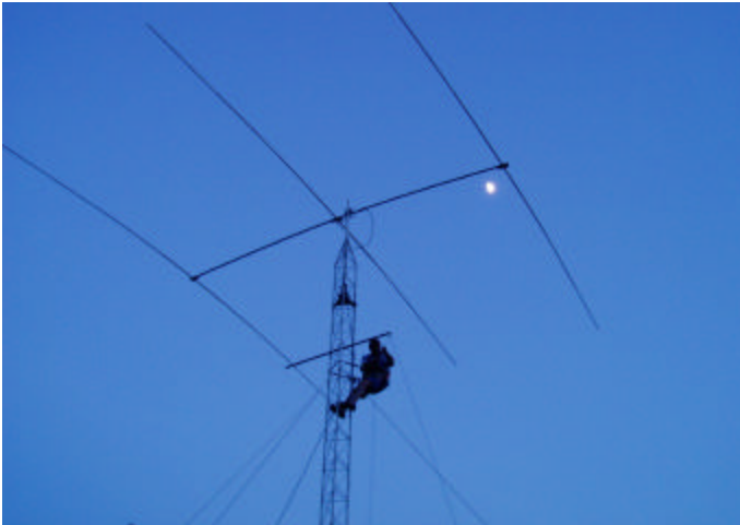
Ken Boyd scampers up the 40 foot tower at dusk on Saturday to install the 40/80m dipole “by the light of the silvery moon”.
