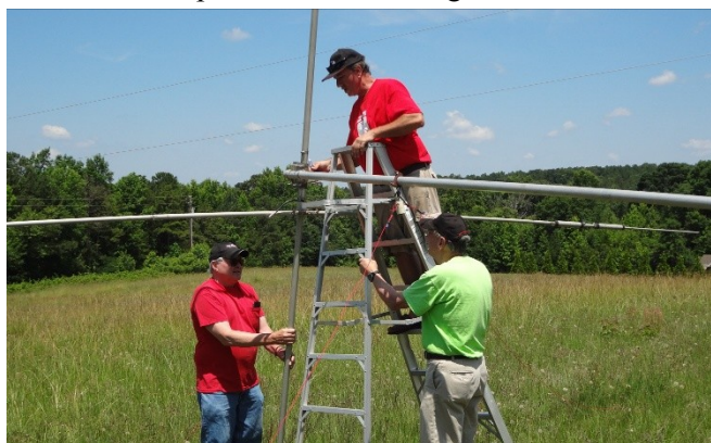
Here are Bill, WW4DD, Joe, KI4TZ, and John, K8YC, installing a tribander on a tilt over tower during the work day the Saturday before Field Day. The red wire between Bill and John is a dipole for 40. We were testing the theory that red dipoles work better than black or white ones.
